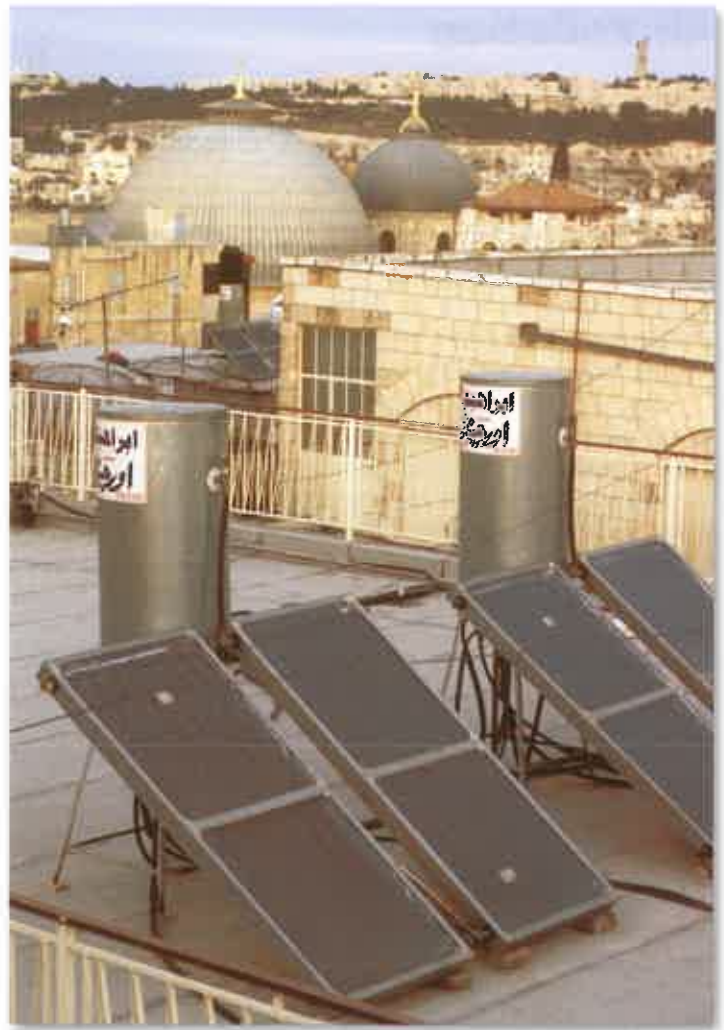
▲ FIGURE 11-56 SOLAR PANELS Solar panels installed on apartment rooftops in the Old City of Jerusalem are used to heat water, which is stored in the adjacent tanks. The domes are the Church of the Holy Sepulchre, built at the site where Jesus is believed to have been crucified, buried, and resurrected (see Chapter 6).
